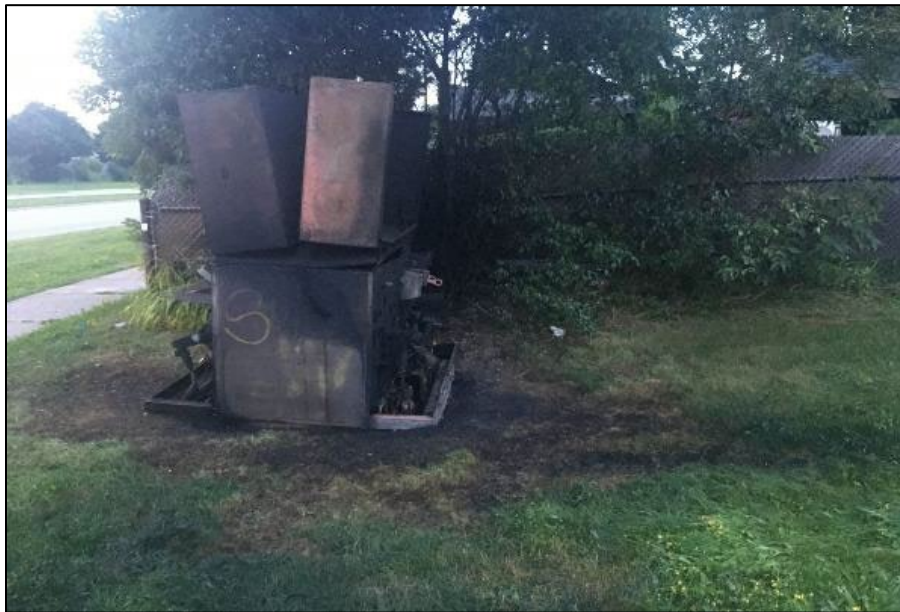
Figure 5.3.3 - 8 Failed Oil-Filled Switchgear
