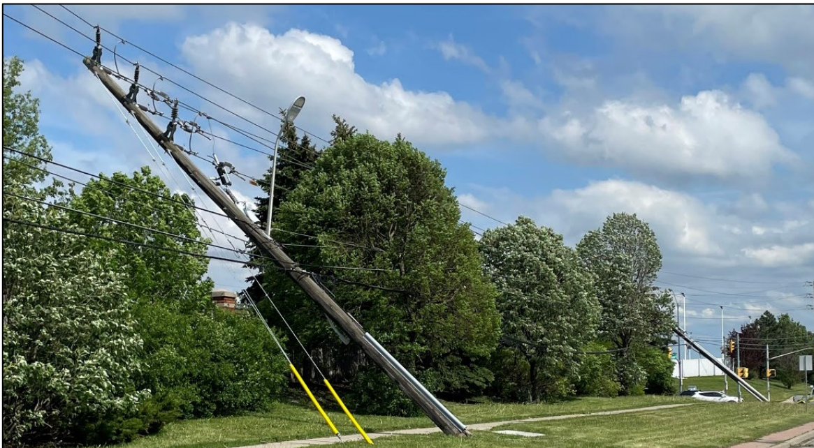
Figure 5.3.2 - 55 Fallen Pole Line Caused by High Winds in Brampton, May 2022
