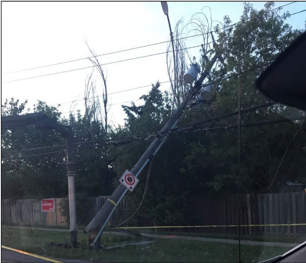
Figure 5.3.2 - 56 Pole Damage Caused by High Winds in Brampton, May 2022
