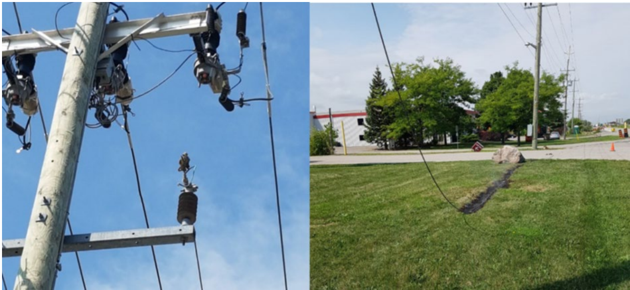
Figure 5.3.3 - 10 Hamilton – Fallen Undersized Wire
