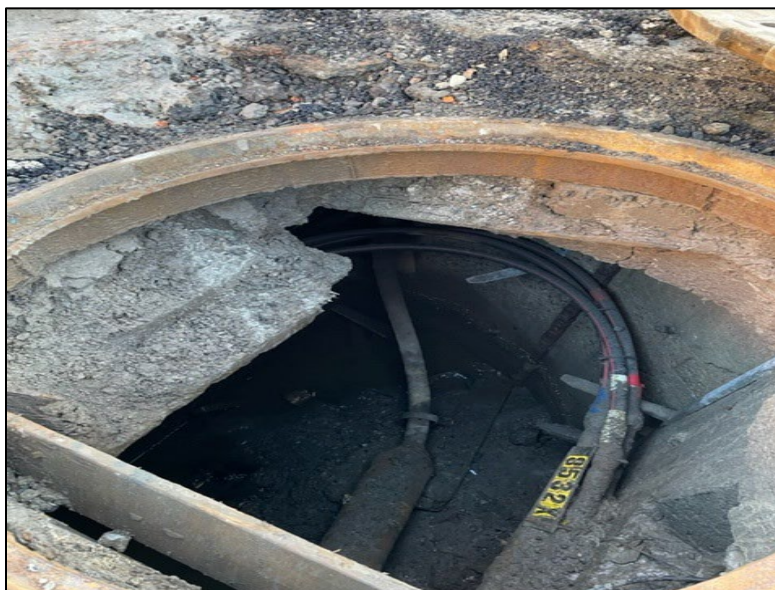
8 9 Figure 5.3.3 - 15 Hamilton – Cable Chamber Roof Collapse
