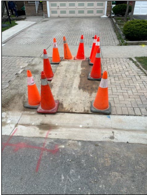
Figure 5.3.3 - 13 Cable Under Driveway
