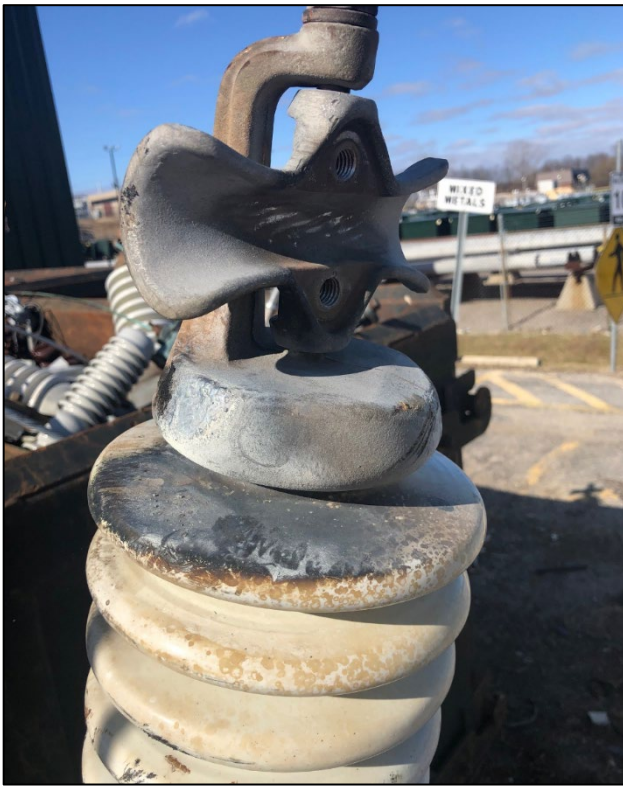
Figure 5.3.3 - 16 Pole Fire Due to Insulator Tracking
