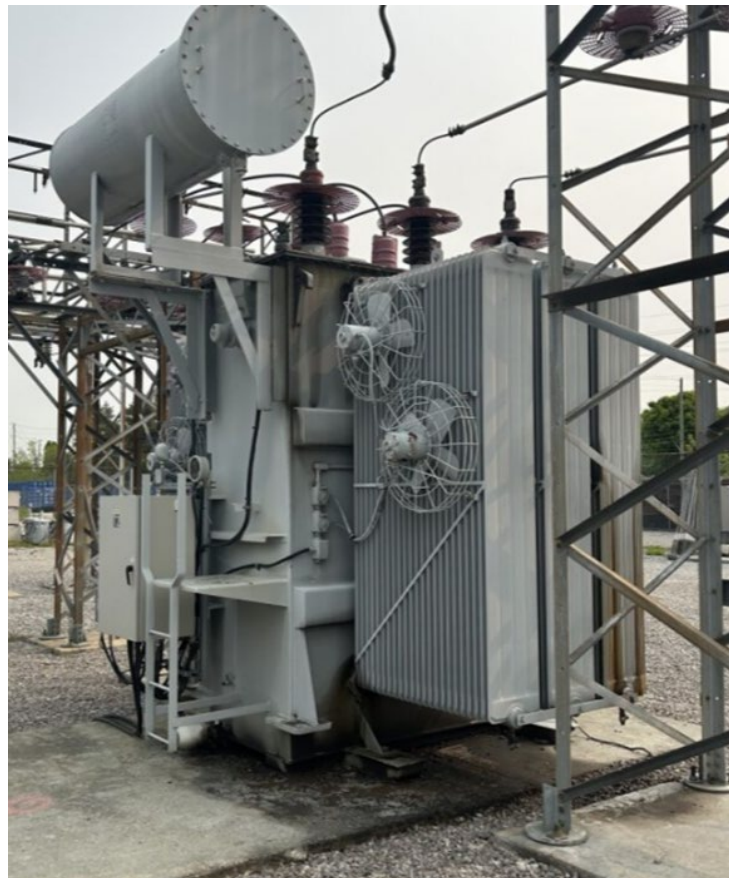
Figure 5.3.2 - 74 Power Transformer Experiencing an Oil Leak
