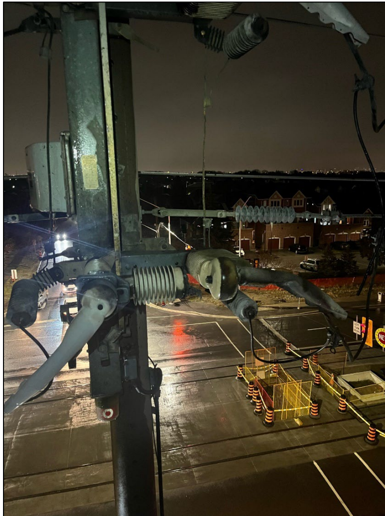
Figure 5.3.2 - 40 Mississauga – Flash Marks on Switch
