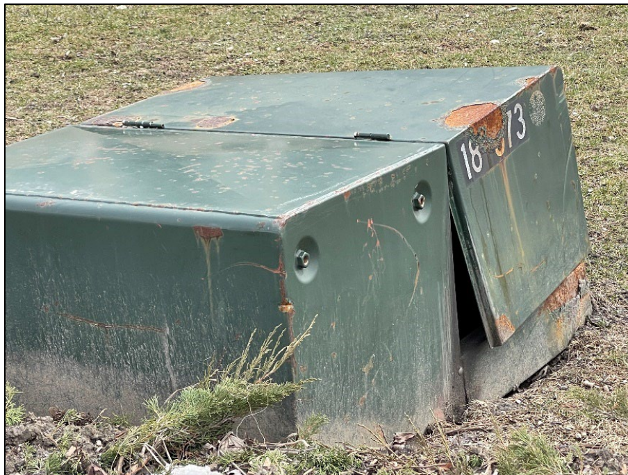
Figure 5.3.3 - 5 Compromised Transformer Enclosure Posing Public Safety Risk
