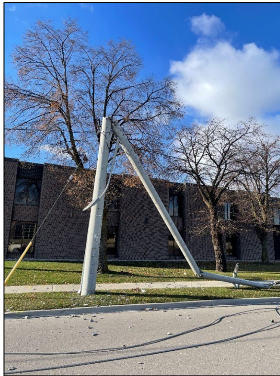
Figure 5.3.2 - 54 Damaged and Fallen Concrete Pole in Mississauga, December 2024
